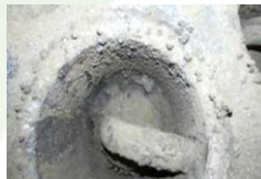
Boiler Ignition Difficulty
