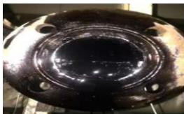
Fuel Line Blockage
